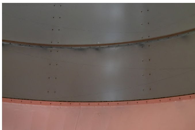
The cone inside fertiliser silos is painted to protect from corrosion and to help empty fertiliser out of the silo.
