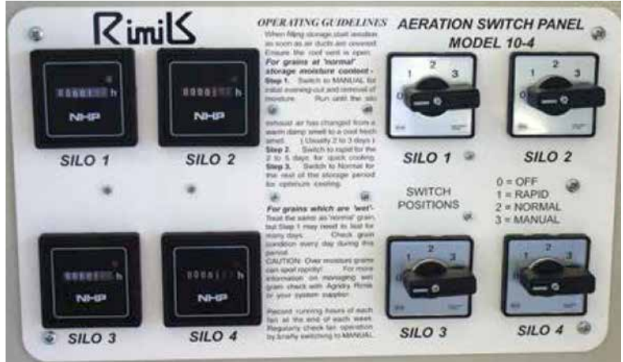
Photo 14: Automatic aeration controllers are the most effective way to cool grain and are designed to manage many storages, from one central control unit.
