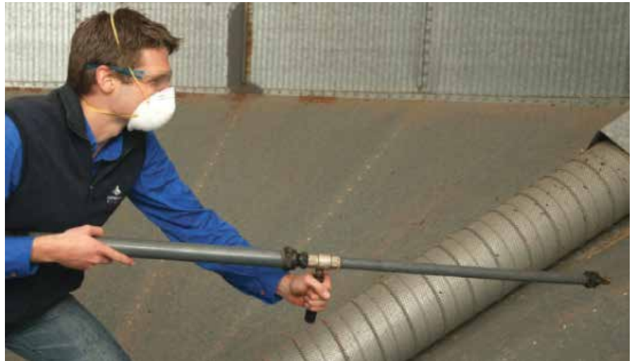
Photo 7: Clean silos, including the silo wall, with air or water to provide a residue-free surface to apply structural treatments.
