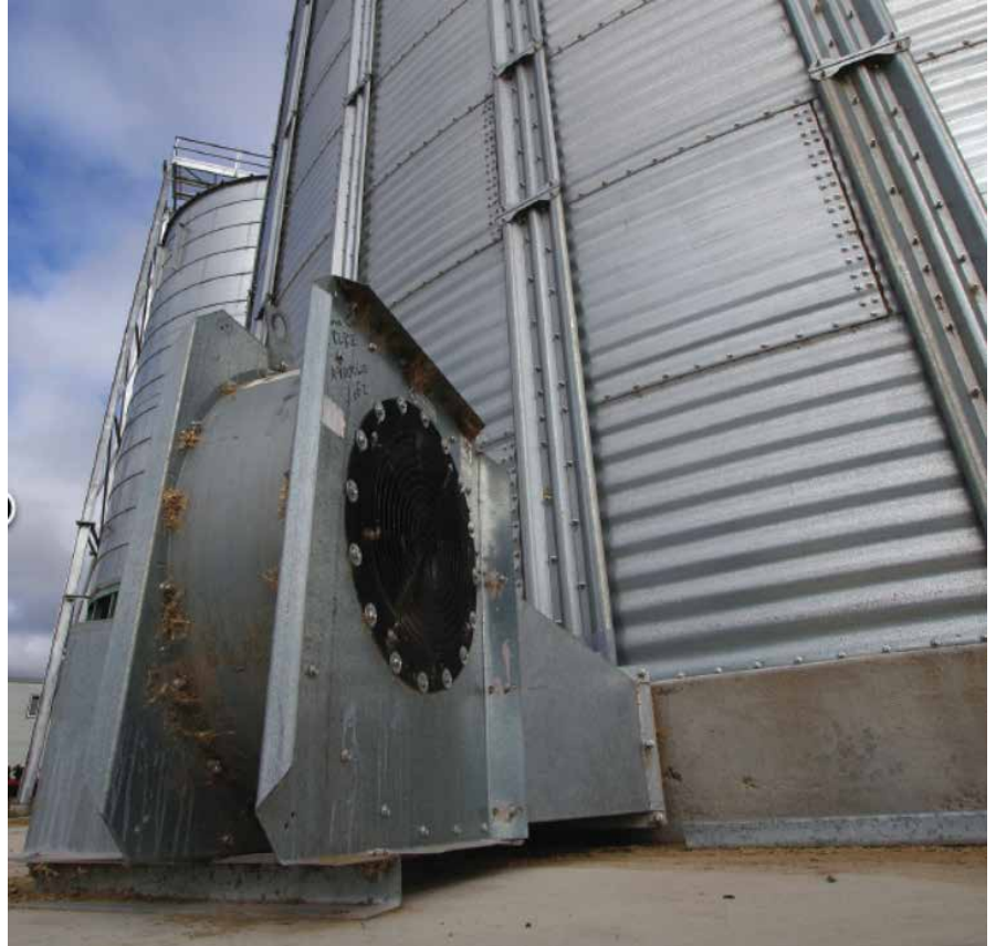
Photo 11: Aeration drying requires careful management, high airflow rates, well designed ducting, exhaust vents and warm, dry weather.
