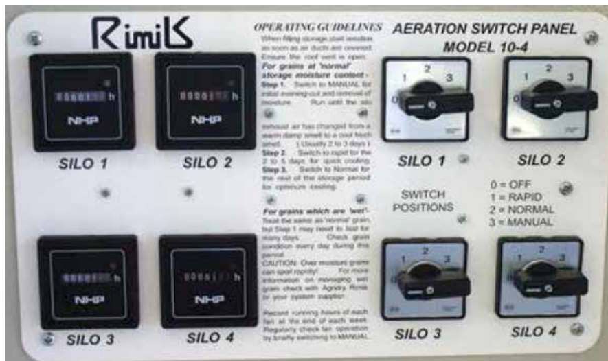
Photo 12: Automatic aeration controllers are the most effective way to cool grain and are designed to manage many storages from a central control unit.
