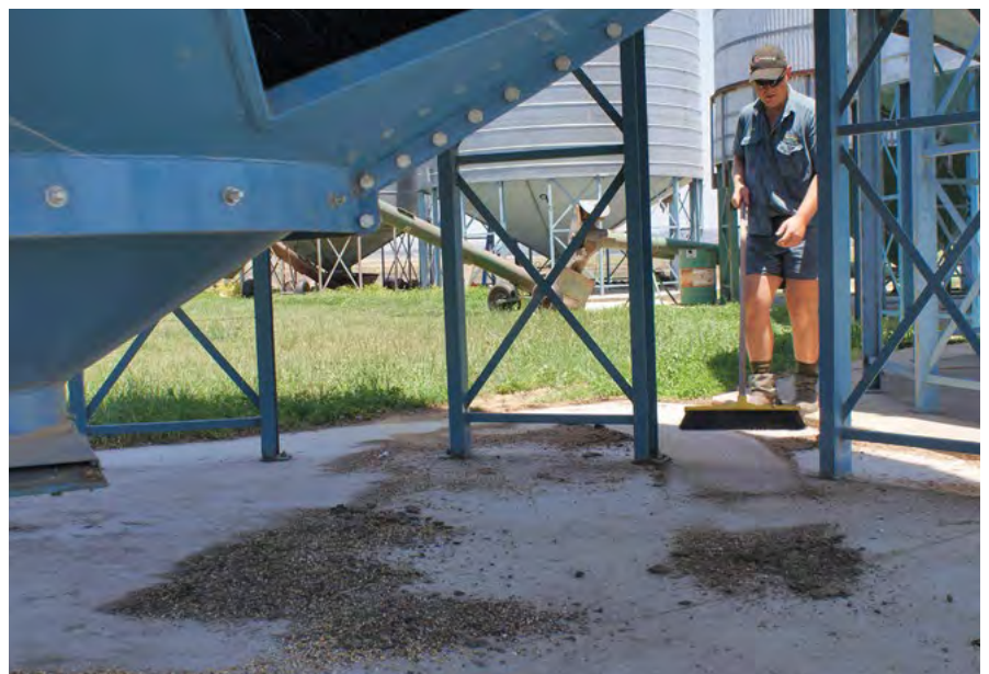
Photo 2: A concrete slab under silos makes cleaning easier. (Source: Chris Warrick, Primary Business)
