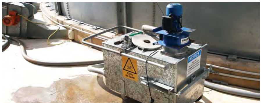
Photo 10: Powered recirculation improves gas distribution through the silo enabling 7-10 day exposure rather than 20 day exposure when fumigating silos greater than 300t capacity. (Source: Chris Warrick, Primary Business)
