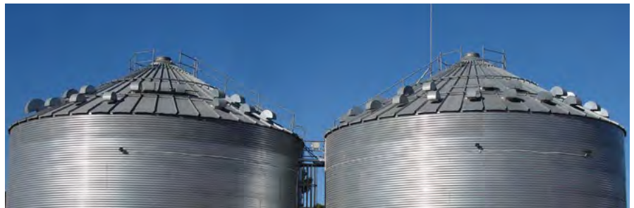
Photo 3: Because aeration drying requires high airflow, extra ventilation is needed to allow air and moisture to escape the silo unrestricted. (Source: Chris Newman, DPIRD)
