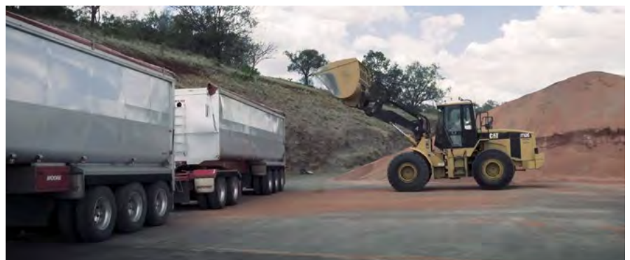
Photo 7: The success of a bunker relies on careful site selection and preparation, quality tarps and equipment for managing tarps and outloading. (Source: GRDC)
