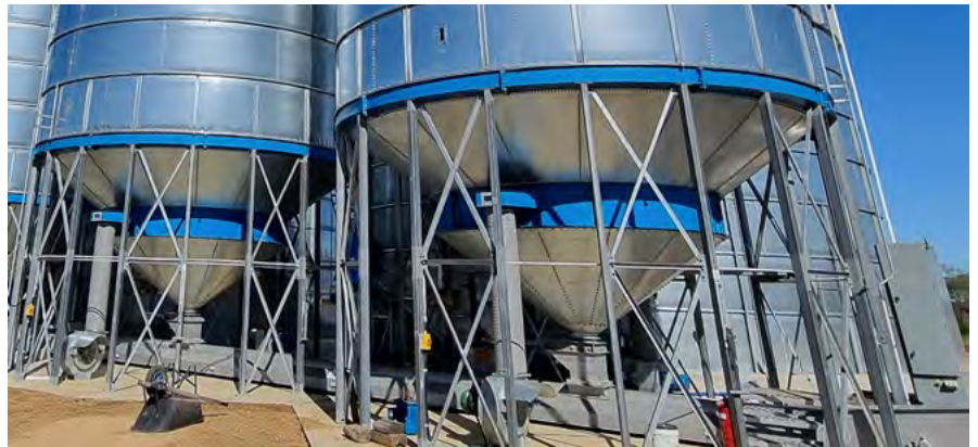
Photo 2: A purpose-built silo for aeration drying has a large fan capable of more than 15L/s/t with ducting right around the silo cone. (Source: Alex Conway)
