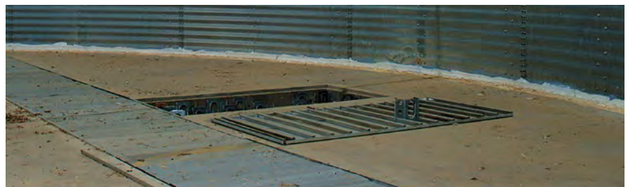
Photo 6: In-floor aeration ducting in flat-bottom silos, which can be removed for cleaning, is ideal. (Source: Ben White, Kondinin Group)
