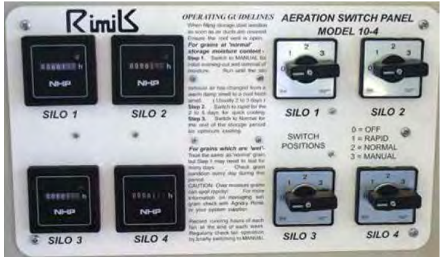
Photo 14: Automatic aeration controllers are the most effective way to cool grain and are designed to manage many storages, from one central control unit.
