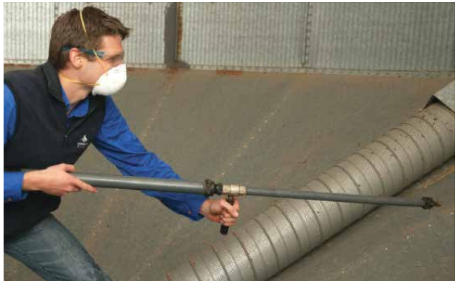
Photo 7: Clean silos, including the silo wall, with air or water to provide a residue-free surface to apply structural treatments.
