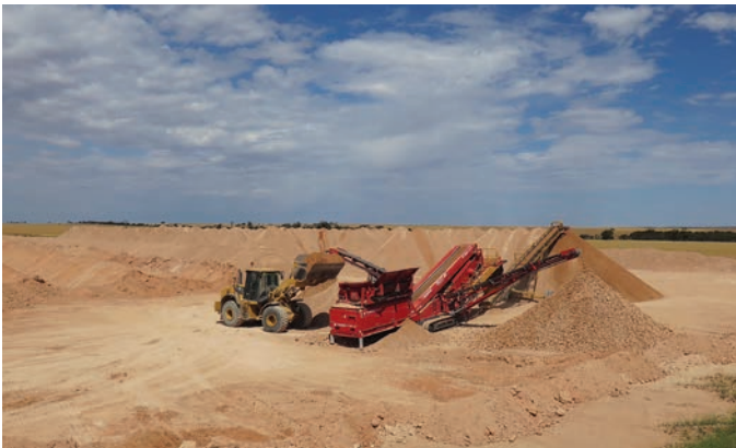
On-farm lime excavation and stockpiling at Kalannie, WA. PHOTO: THE LIEBE GROUP
