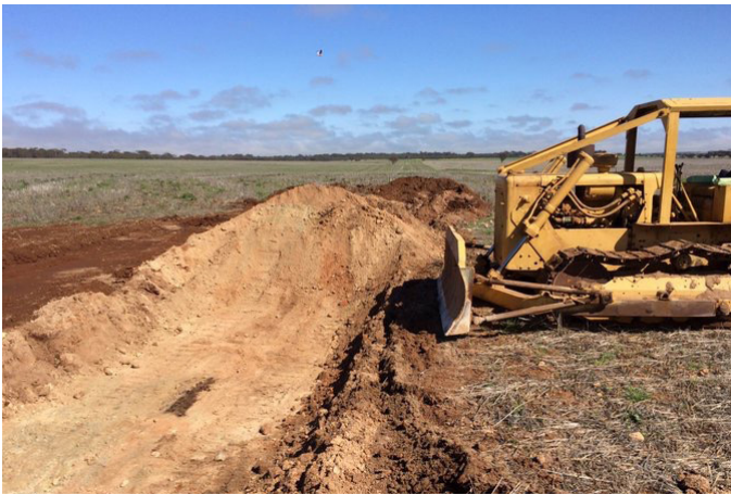
Extracting on-farm lime near Narembeem, WA. The source is first pushed up in shallow runs with a bulldozer. PHOTO: MAP IQ
