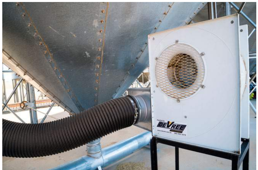
Photo 4: Silo fitted with aeration fan for cooling.
