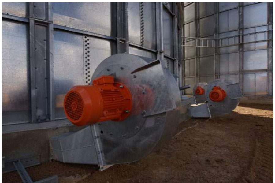
Photo 5: Aeration drying requires air-flow rates of 15–25 L/sec/tonne of grain.
