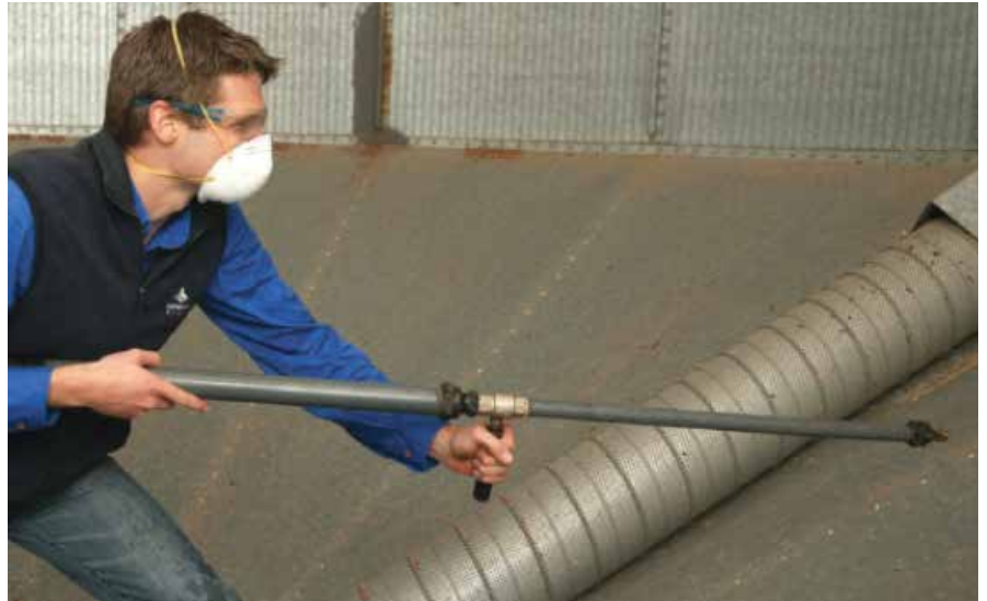
Figure 6: Clean silos, including the silo wall, with air and/or water to provide a residue-free surface to apply structural treatments.
