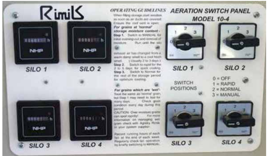
Figure 12: Automatic aeration controllers are the most effective way to cool grain and are designed to manage many storages, from one central control unit.
