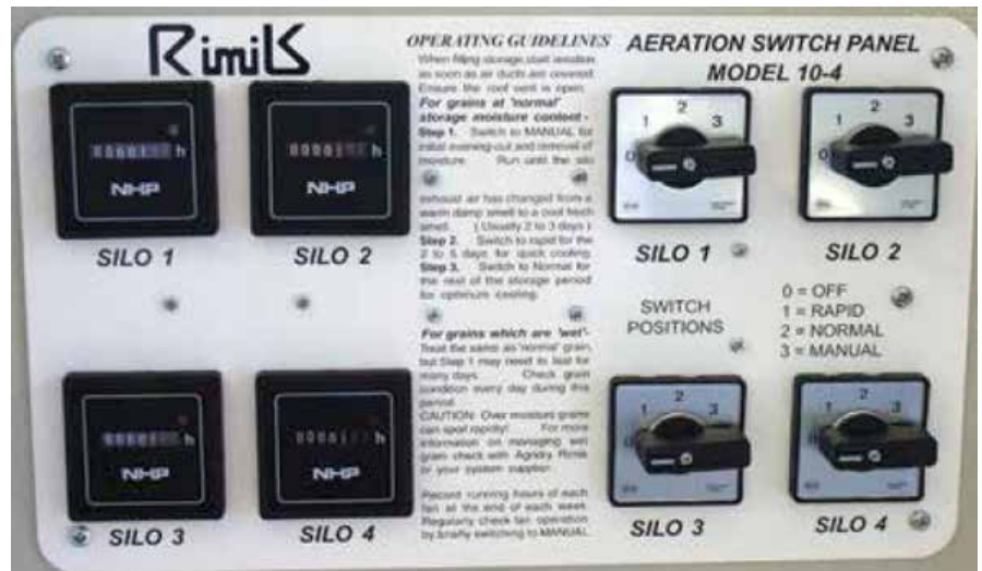
Photo 9: Automatic aeration controllers are the most effective way to cool grain and are designed to manage many storages, from one central control unit.
