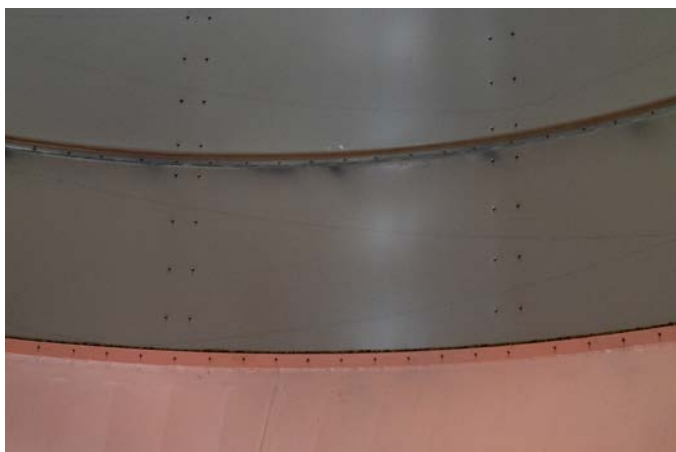
The cone inside fertiliser silos is painted to protect from corrosion and to help empty fertiliser out of the silo.
