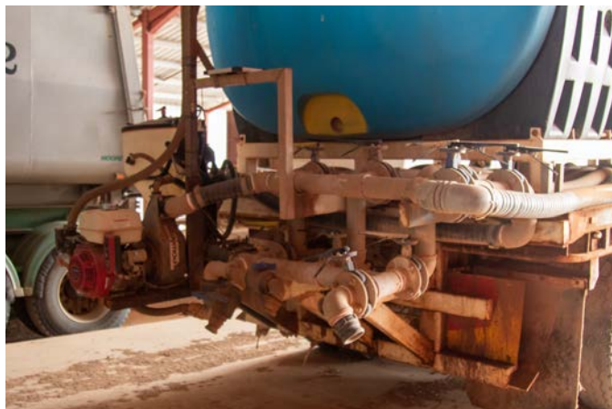
The plumbing system on the semitrailer, which contains three 15,000L tanks, allows for product mixing in the tanks (that is, the addition of trace elements) and it can fill the nurse trucks from either side. Photo: Petrina Ronald
