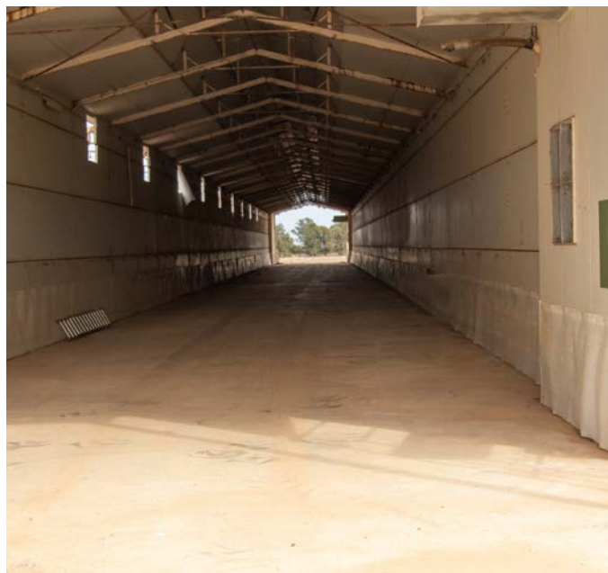
The chook shed was gutted and holes added along one side so fertiliser can be augered into the shed, which has the capacity to store 700t of urea and 1000t of MAP.
