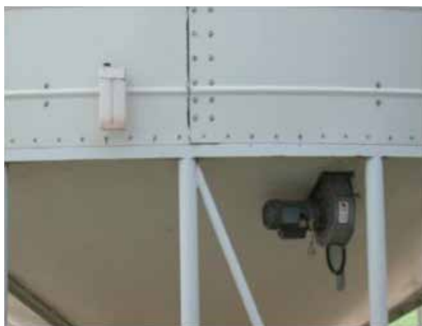
Figure 1: Standard aeration cooling fan. (Photo: Australian Oilseeds Federation)
